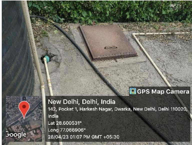
Underground Water Tank
