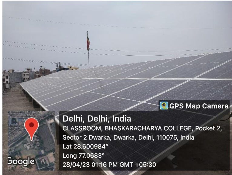
Solar Power Plant
