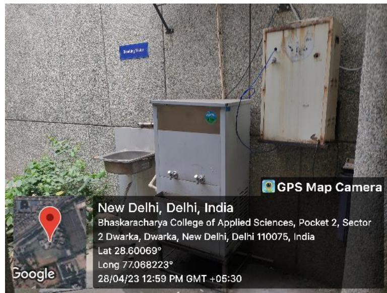
Water Cooler for drinking water
