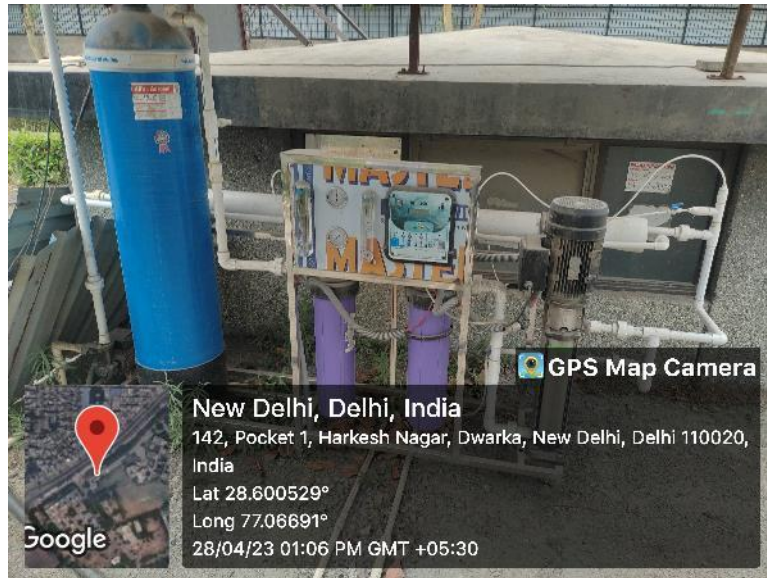
RO Plant at terrace
