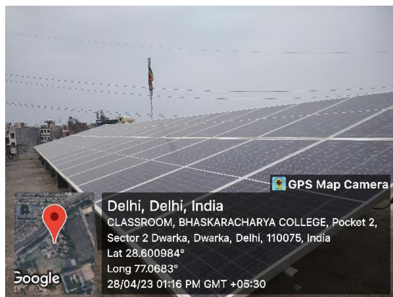
Solar Power Plant
